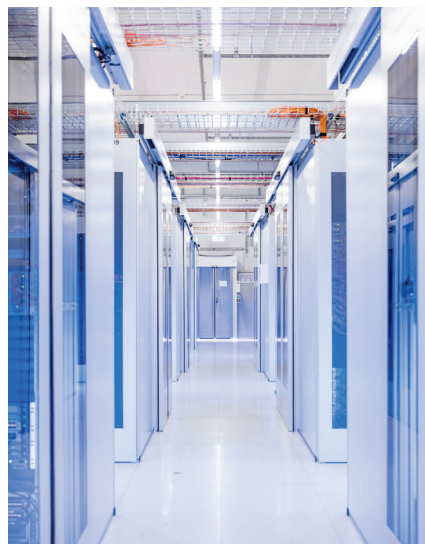
Banks find added value in commercial data centres where lots of partners, connections and entire ecosystems come together.
